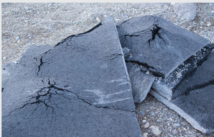
Figure 16-1: Asphalt containing asbestos
